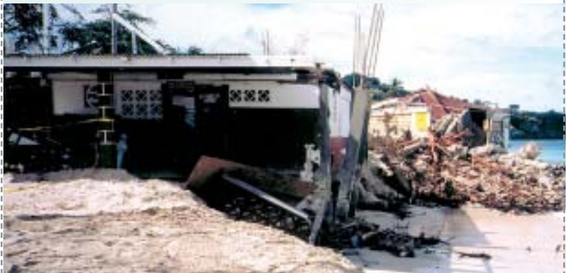
Much of this same building was reduced to rubble by Hurricane Lenny in 1999
